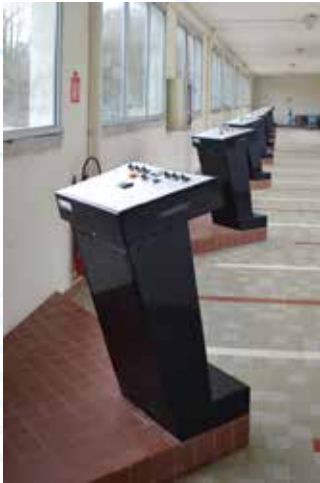
Before: Manual control of facilities
